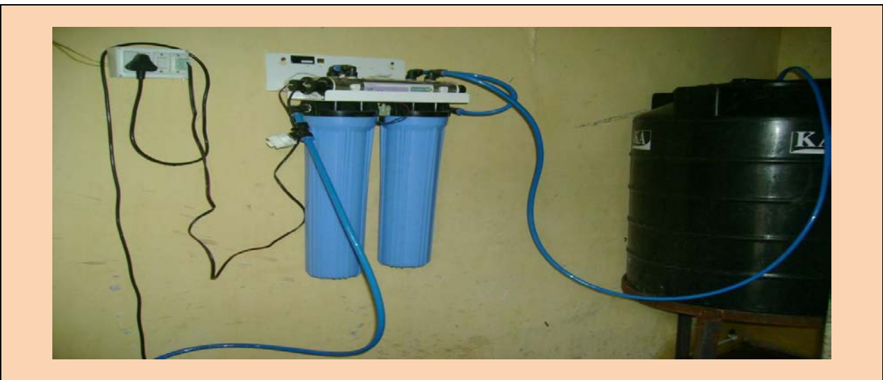
(Potable and safe drinking water – Primary school, Magnad)
